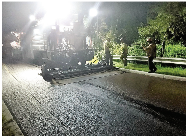
Pictured: Slurry Seal treatment being applied to the Route 33, CR 527 to Howell Road Pavement Preservation Project in Monmouth County.
