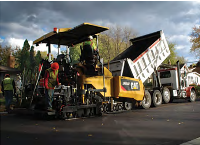
Crews working for SJ Gas repaving a road in Primrose Gate as required by the Township at no cost to the Winslow.
